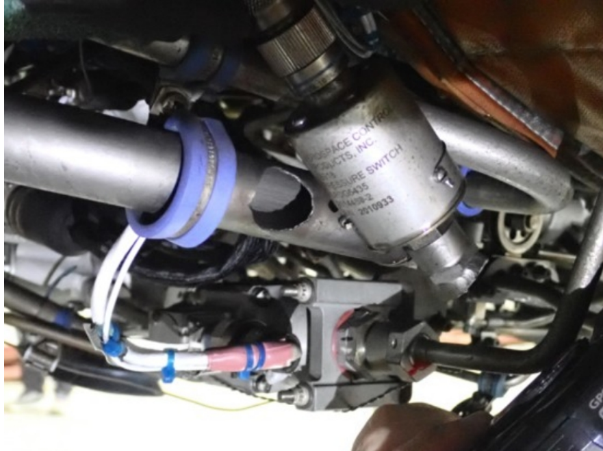
Figure 1. Right engine fuel tube assembly and fuel pressure switch
